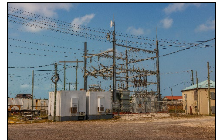
Belize City Substation at Magazine Road
