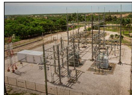
Westlake Substation at Mile 8 George Price Highway
